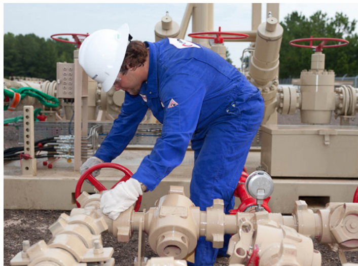
Plug valve choke manifolds regulate downstream pressure and volume accurately.
