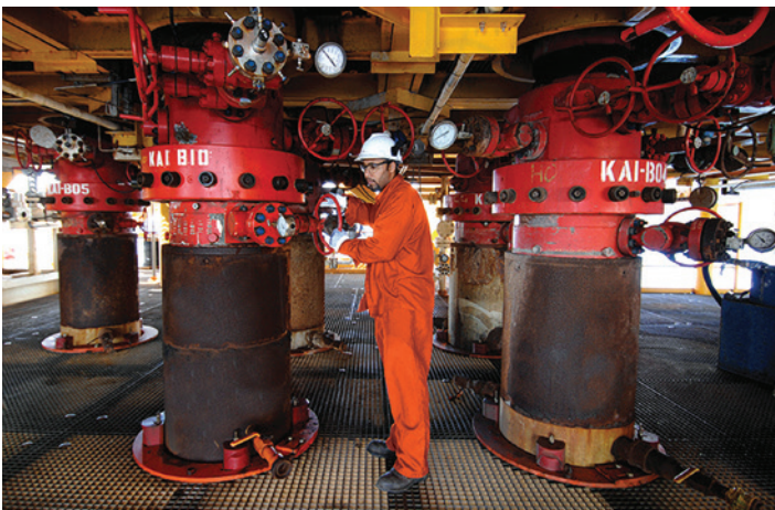
A qualified Cameron technician monitors wellhead performance.
