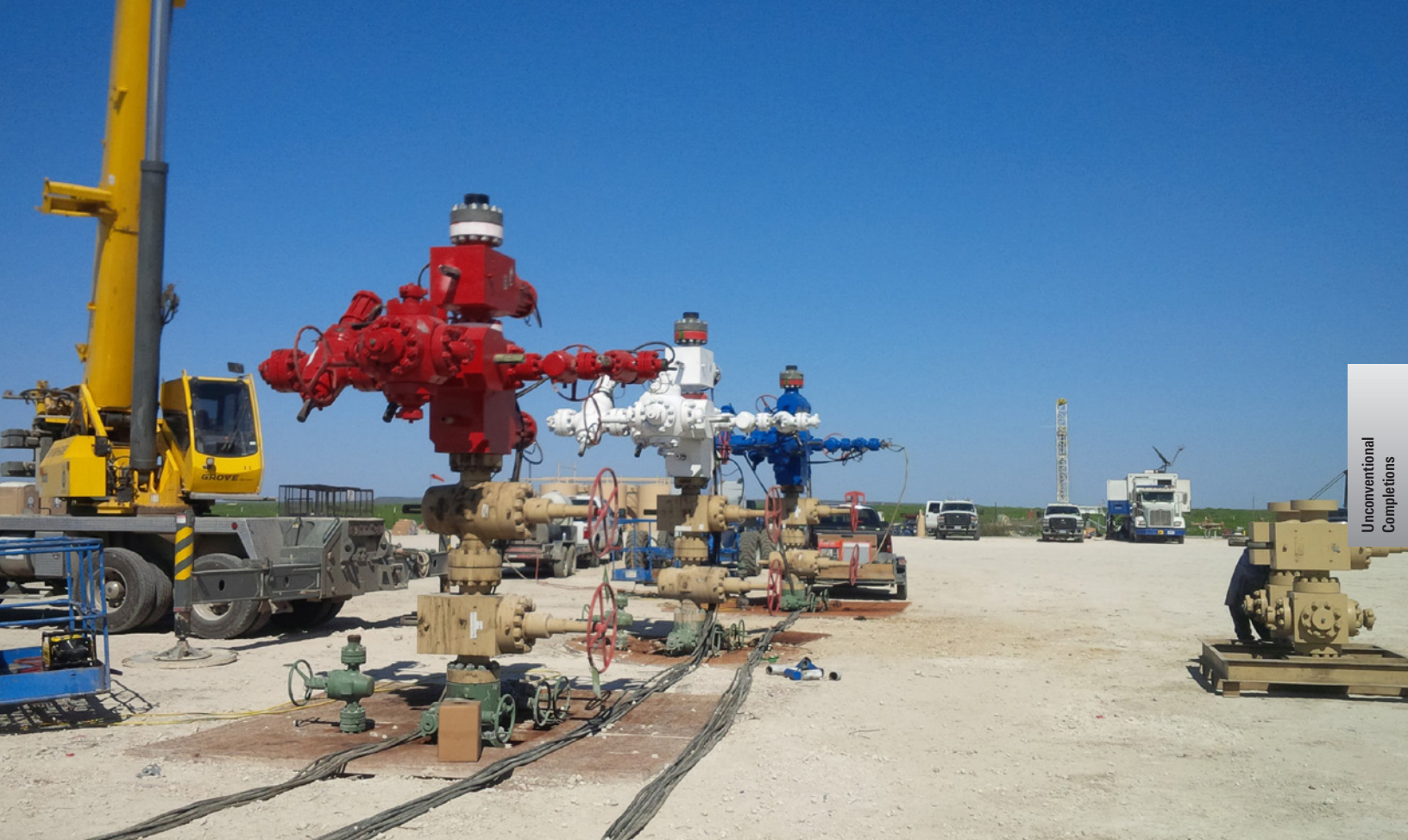
The composite frac tree's reduced height decreases the bending stress transferred from the goat head to the tree and wellhead connections below.
