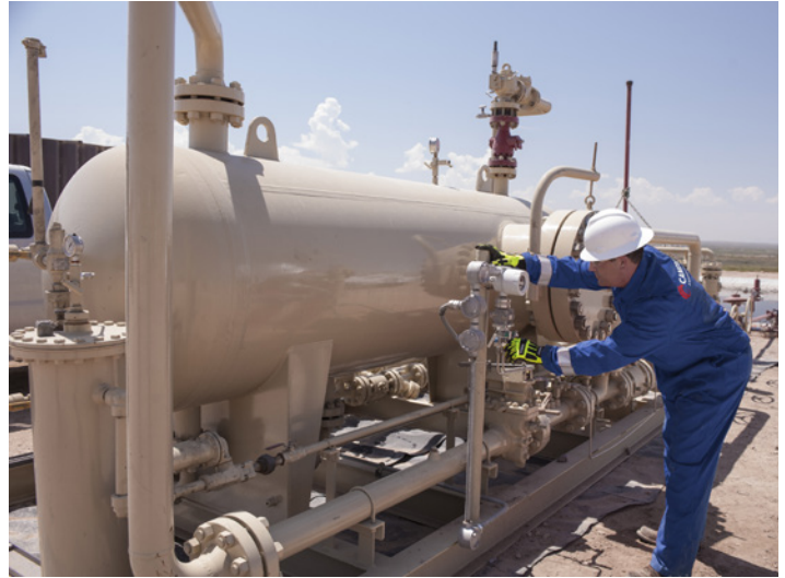
Low- and high-working-pressure vessels are used to separate oil, water, gas, and sometimes solids (sand) into individual streams for more accurate measurement and discharge control.
