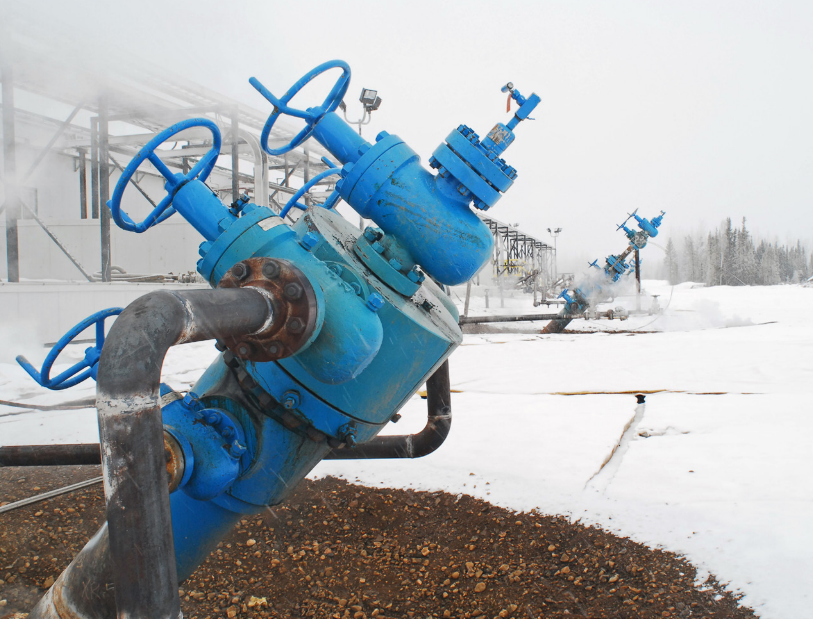
Cameron heavy-oil wellhead systems provide fluid and pressure control for effective recovery.
